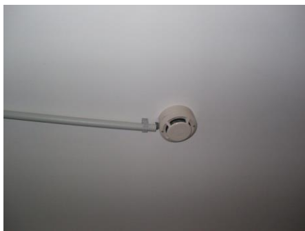
Fig. 3. Fire detection and alarm system.
