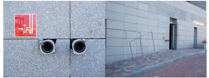
Fig. 4. Standpipes of indoor fire main.
