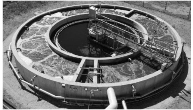
Figure 7. Combined aeration and clarification concentric reservoirs
