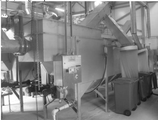
Fig. 4. Pretreatment equipment: mechanical screen and aerated grit separator
