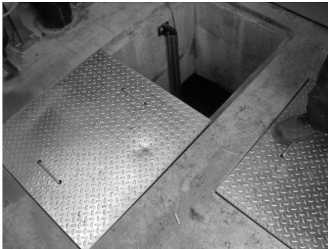
Fig. 3. Sewage intake pumping station manholes
