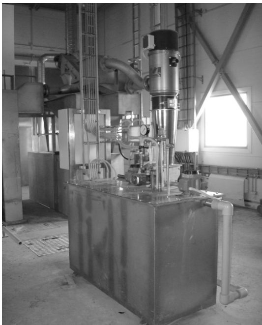
Figure 6. Soda preparation unit with vacuum elevator for dry powder
